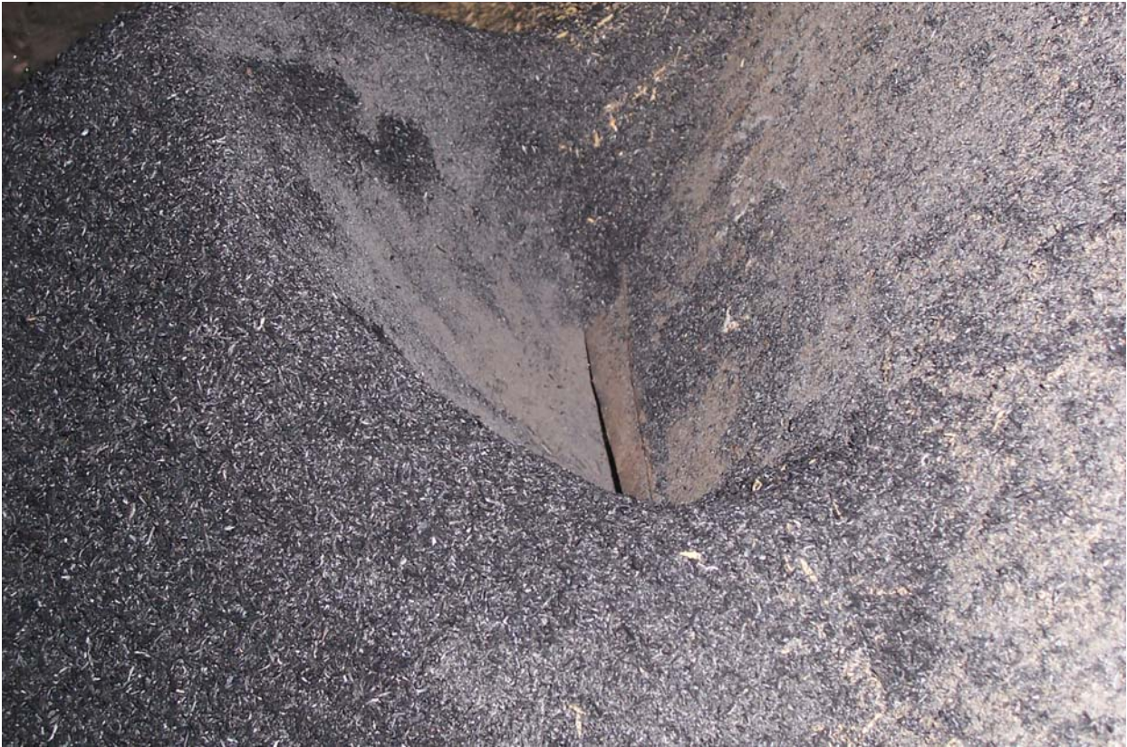
Case study 4: Photo 9- Waterwall roof with leakage
