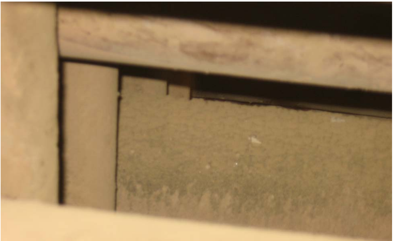
Case study 7- Photo 16: Flue gas condensation as droplets over the ash is seen. A proof air ingress & ash leak.
