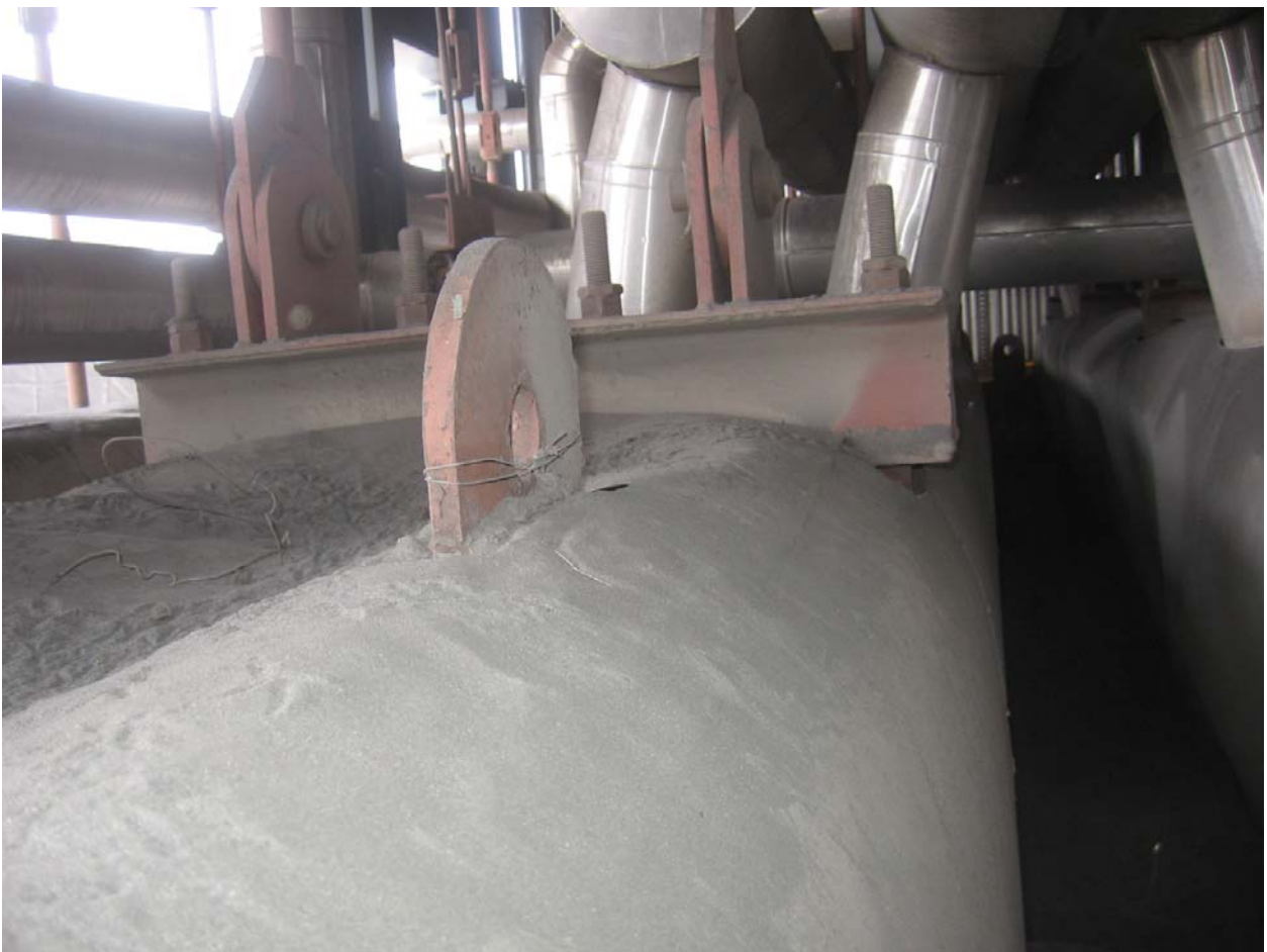
Case study 6- Photo 13- Ash leakage marks at SH header area above the roof in a new boiler.
