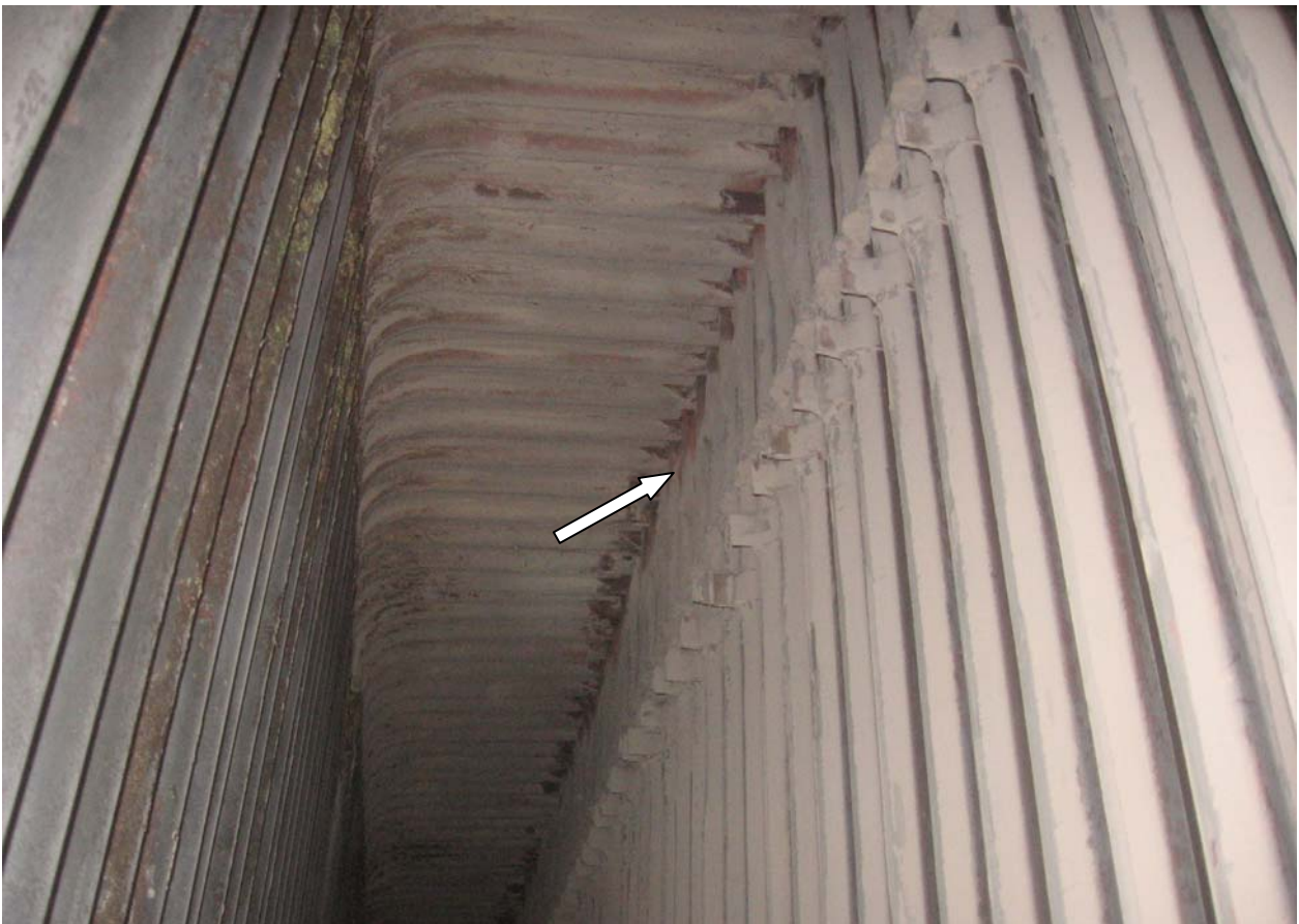
Case study 6-Photo 12: Inside view of SH coil penetrations in the roof shows the air ingress.
