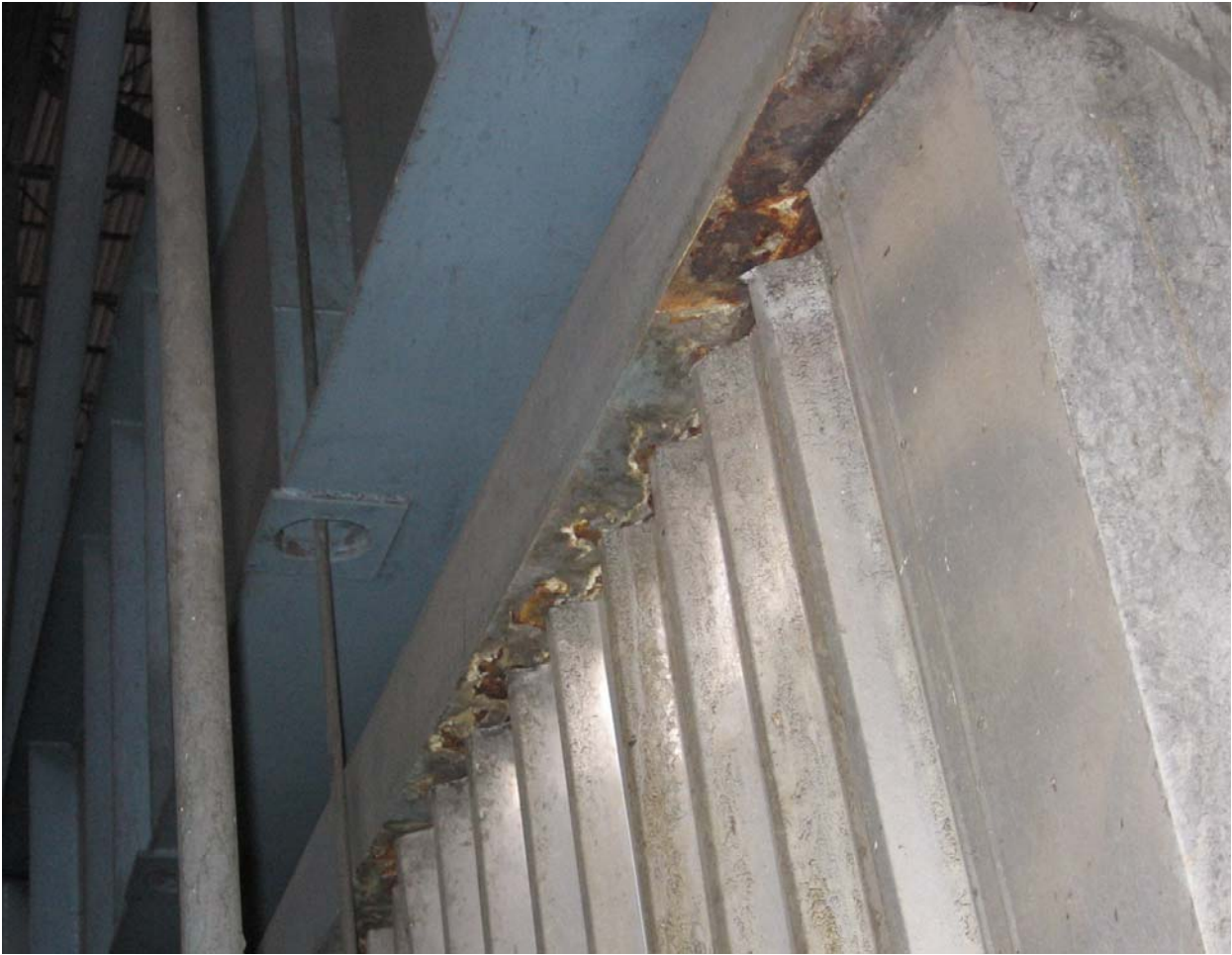
Case study 7- Photo 15- corrosion seen at roof beams – indication of gas leakage. With high sulfur fuel the corrosion damage will be more.
