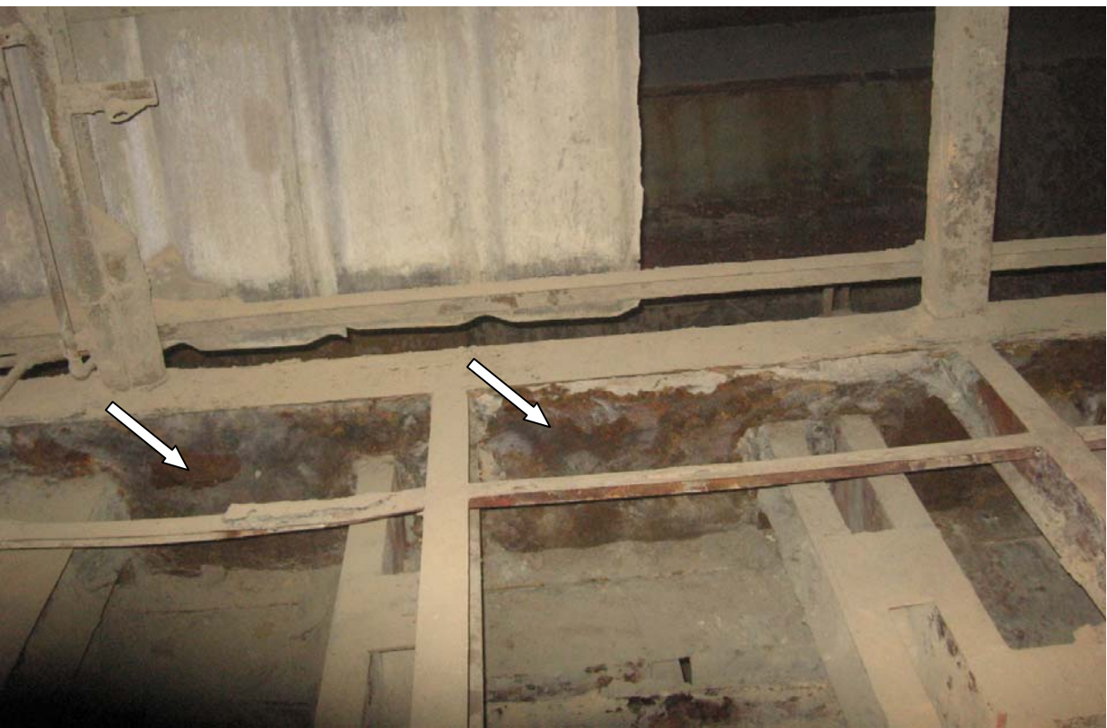
Case study 2: Photo 5- Roof beams under corrosion.
