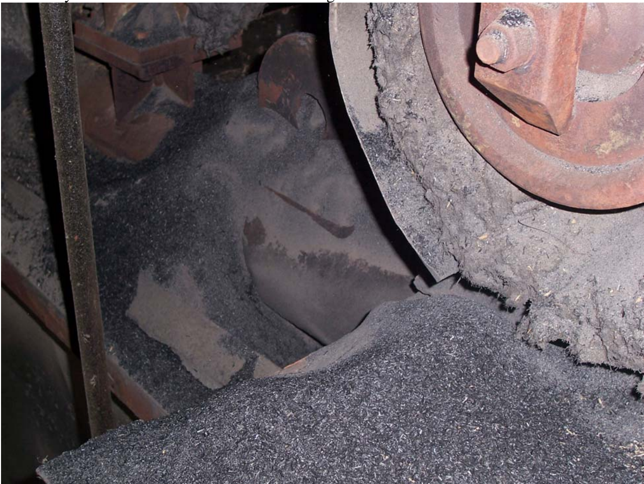
Case study 4- Photo 10: leakages around the headers.
