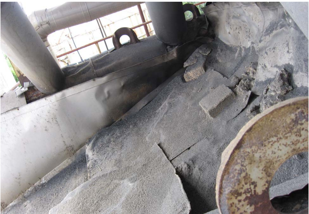
Case study 5 -Photo 11- marks of flue gas leakage.
