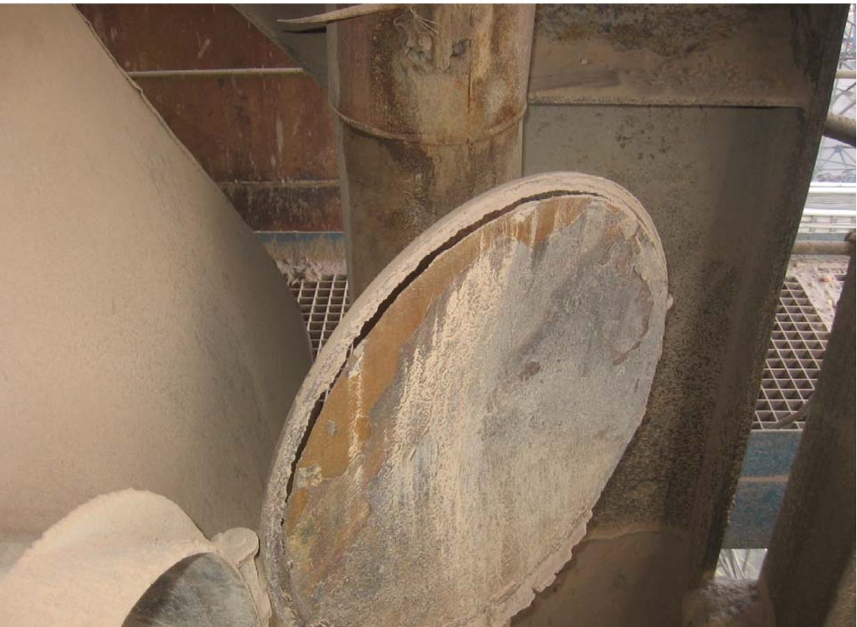
Case study 2: Photo 6: leaky penthouse door.
