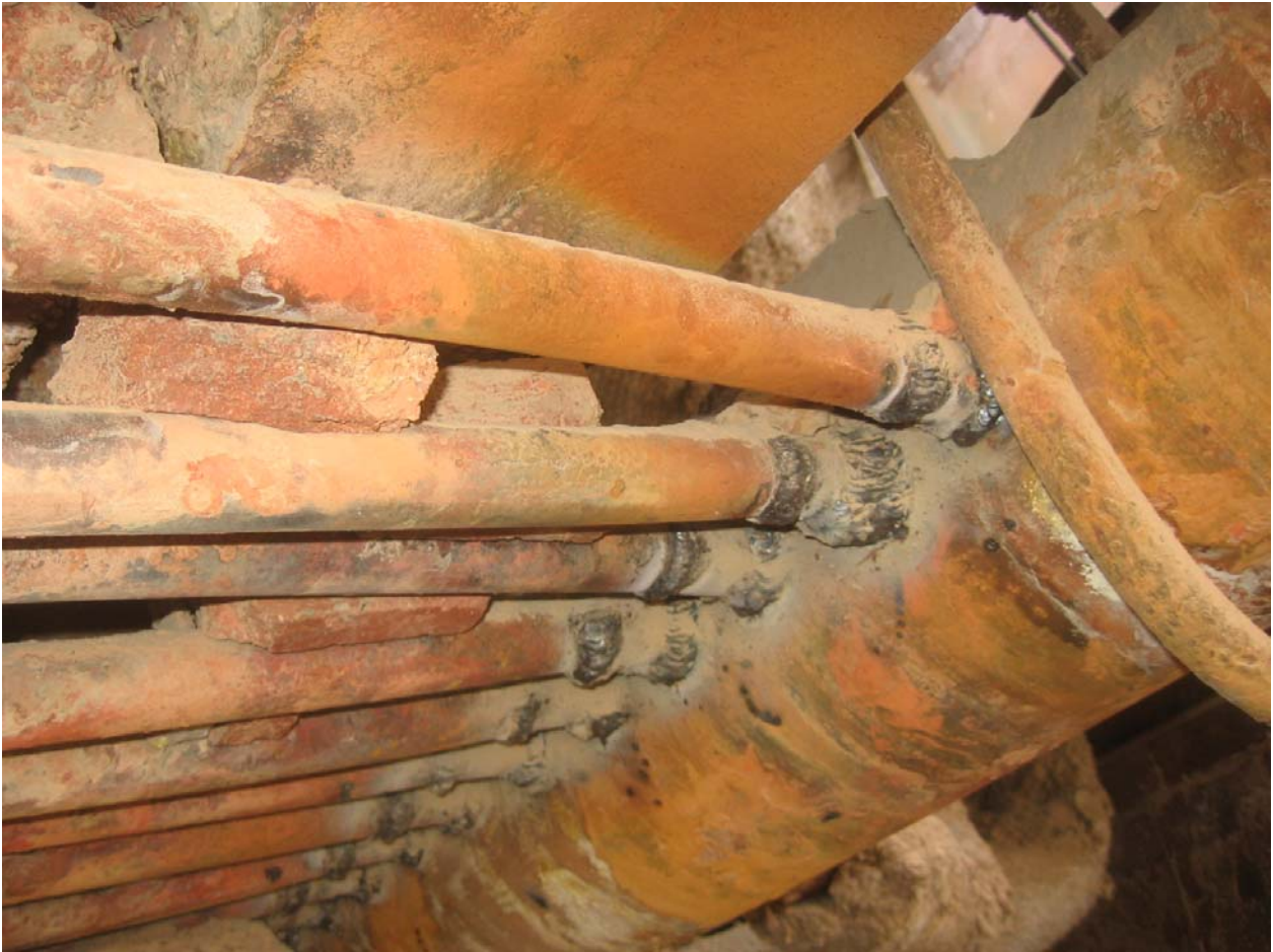
Case study 2- Photo 7-Failures of weld joint of dissimilar materials caused by high steam temperature.
