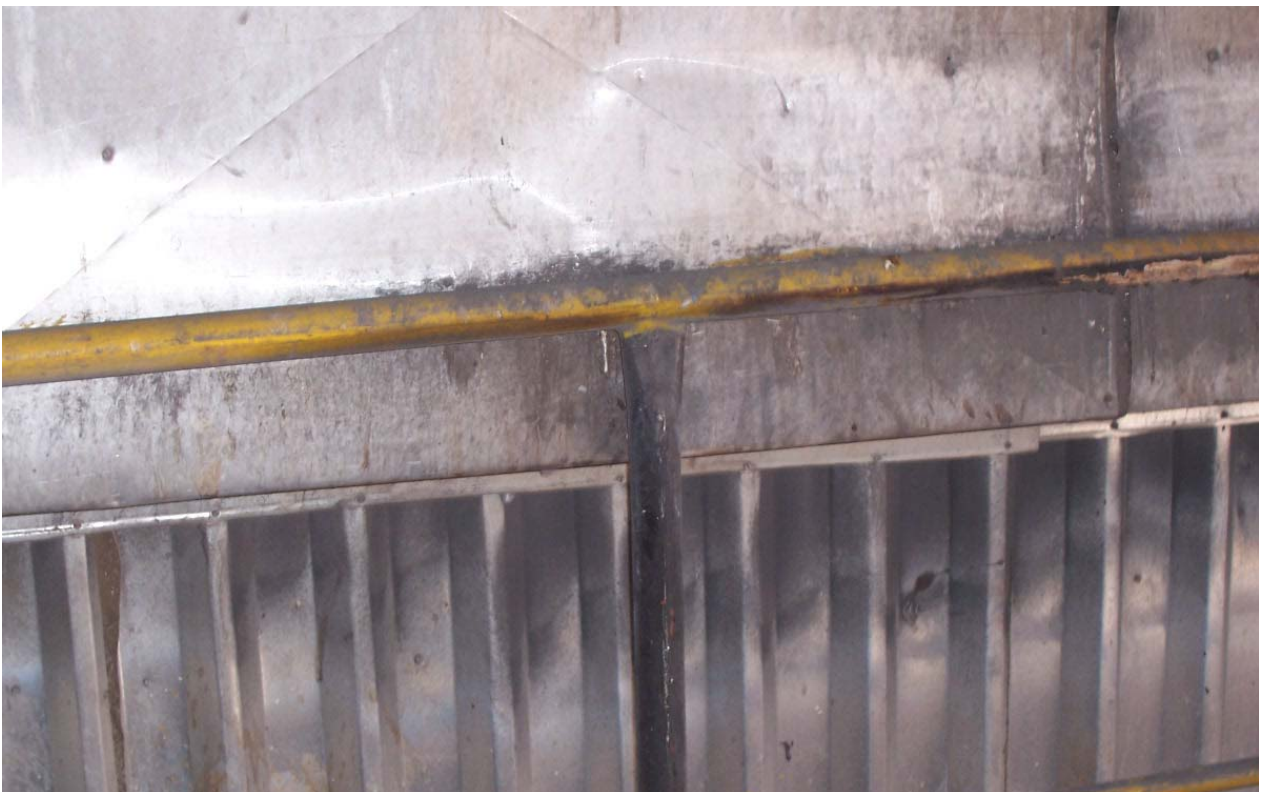
Case study 7 -Photo 14: dust leakage seen around the side cladding sheet below the penthouse.
