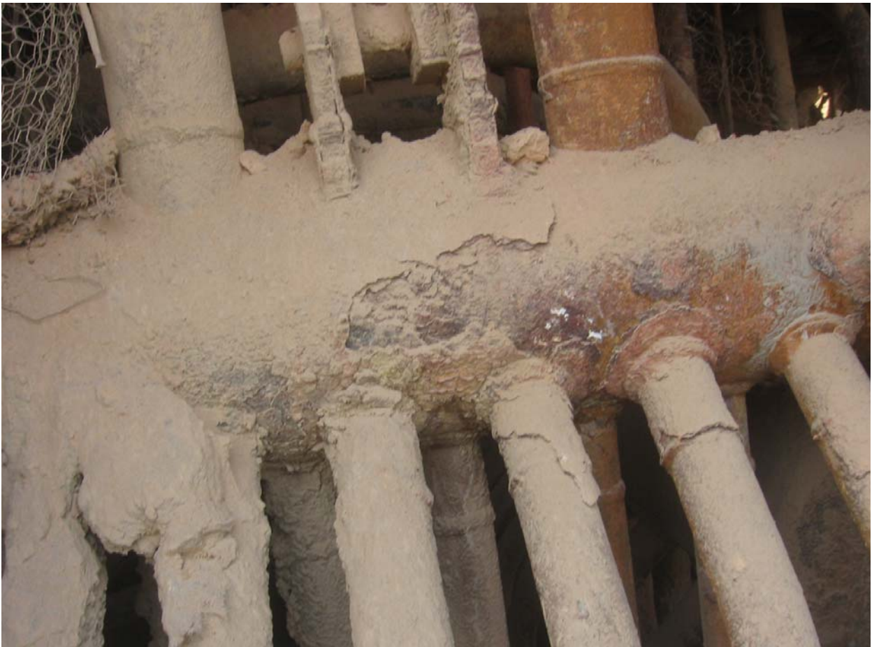
Case study 2: Photo 4: Corroded waterwall header due to condensation of flue gas.
